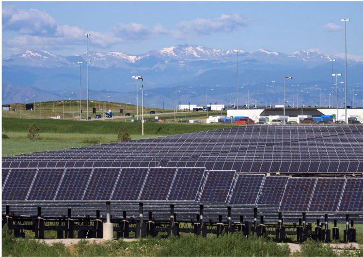
Ground-Mounted PV Example
